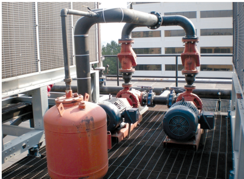
The retrocommissioning process can correct problems such as this: incorrect piping, with the expansion tank on the discharge side of pumps.
