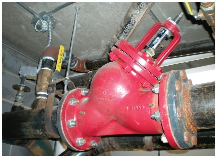
Inspections during the retrocommissioning process can reveal the negative impact of an oversized pump: excessive throttling on the triple-duty valve.
