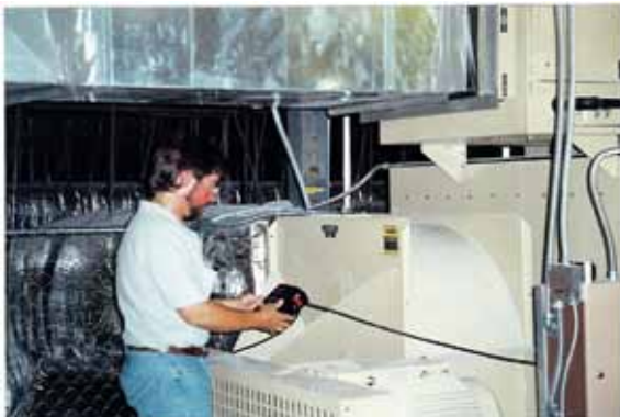
⌘ A technician is measuring fan performance to verify proper building ventilation rates.
